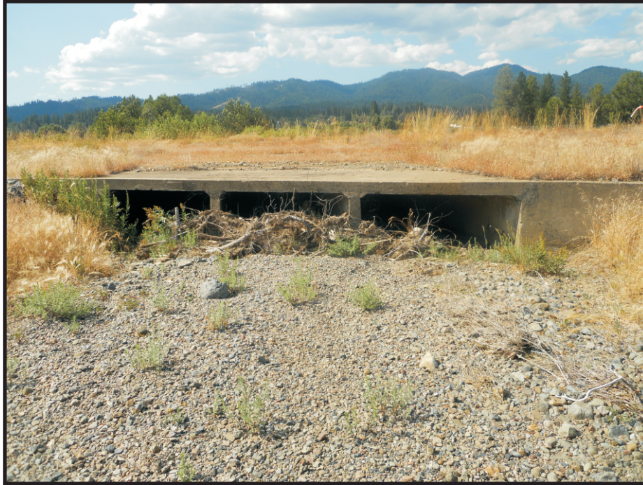
Kingsbury Gulch at 3-box culvert under Runway 7-25. Photo was taken July 2010, looking north.
