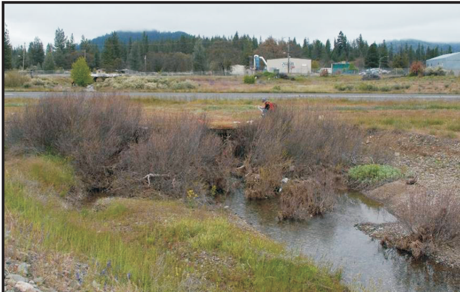
Kingsbury Gulch at 3-box culvert under Runway 7-25. Photo taken May 2010, after a rainfall event. Photo is looking south.
