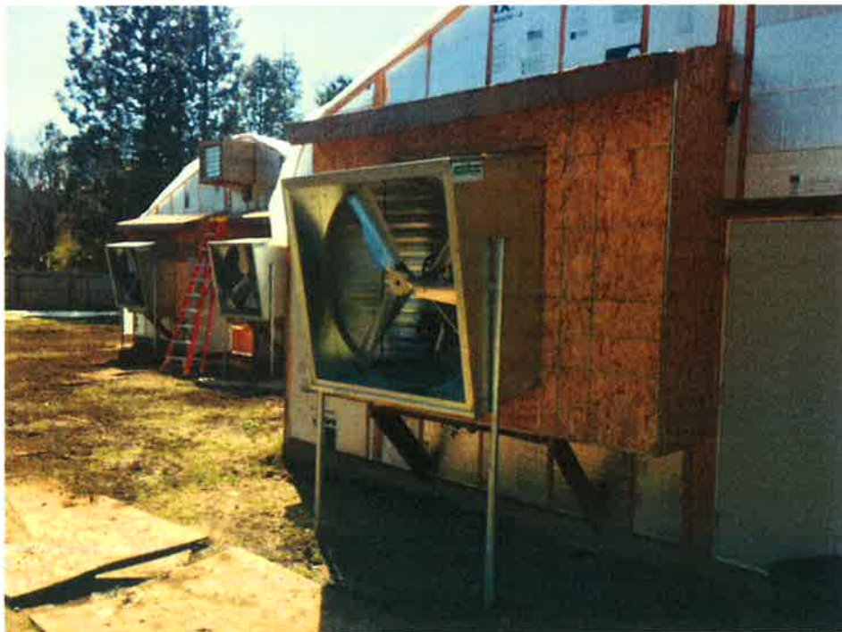
Picture 4: Exterior pictures of two (2) Greenhouses mechanical systems, including distance between existing fence separating cultivation area from APN 017-440-25
