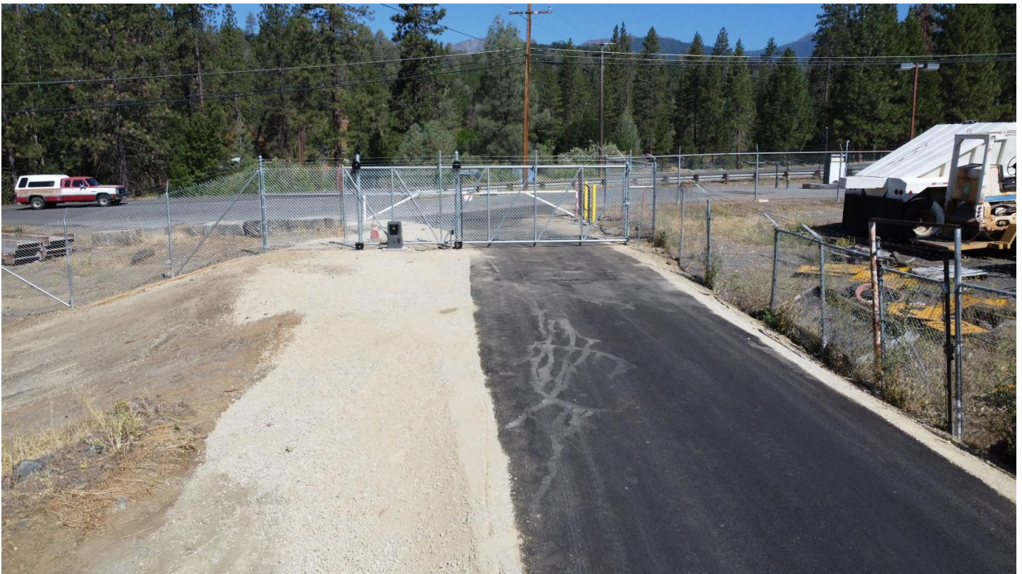
Transit Parking Lot; Completed Fence and Gate at the State Route 3 Entrance (Main Gate)
