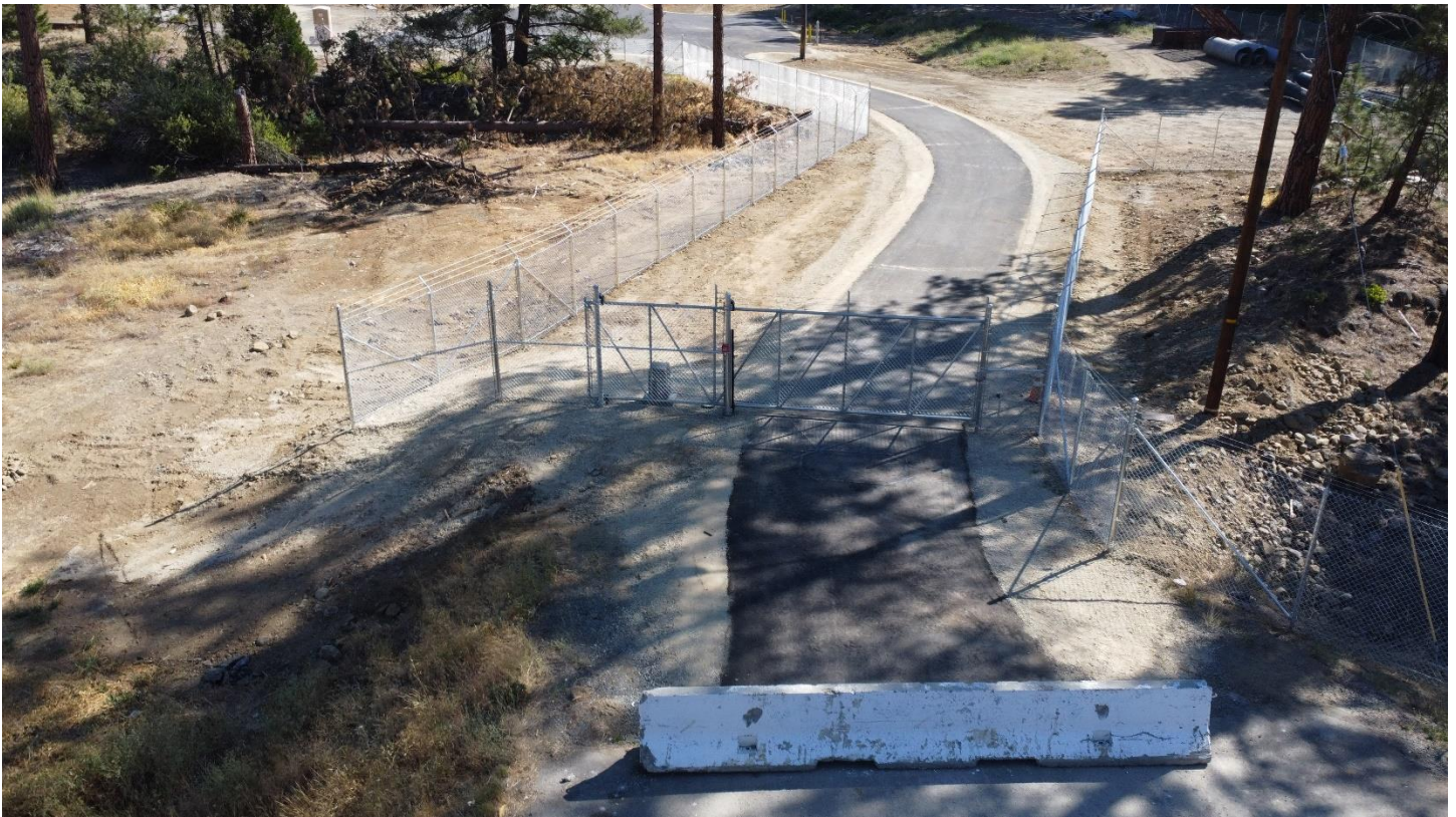
Transit Parking Lot; Completed Fence and Gate at the Lance Gulch Entrance
