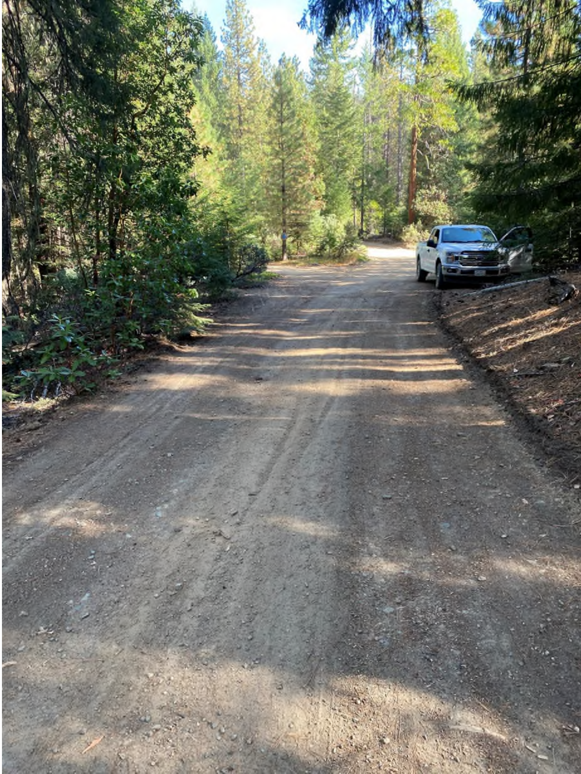
Access road to CCL 106, Mr. Coogan claims these roads have been graded/widened without USFS approval. (photo taken 10/11/2022)
