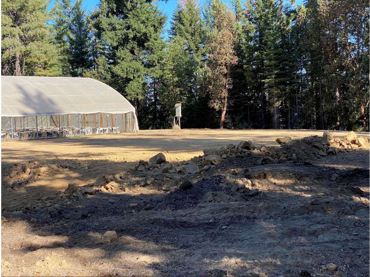
Evidence of grading on Mr. Petkov property (photo taken 10/11/22)
