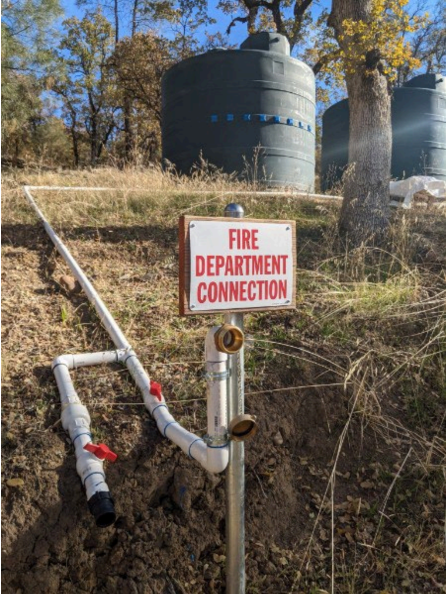
Attachment 10 – Fire Suppression Connection Image
