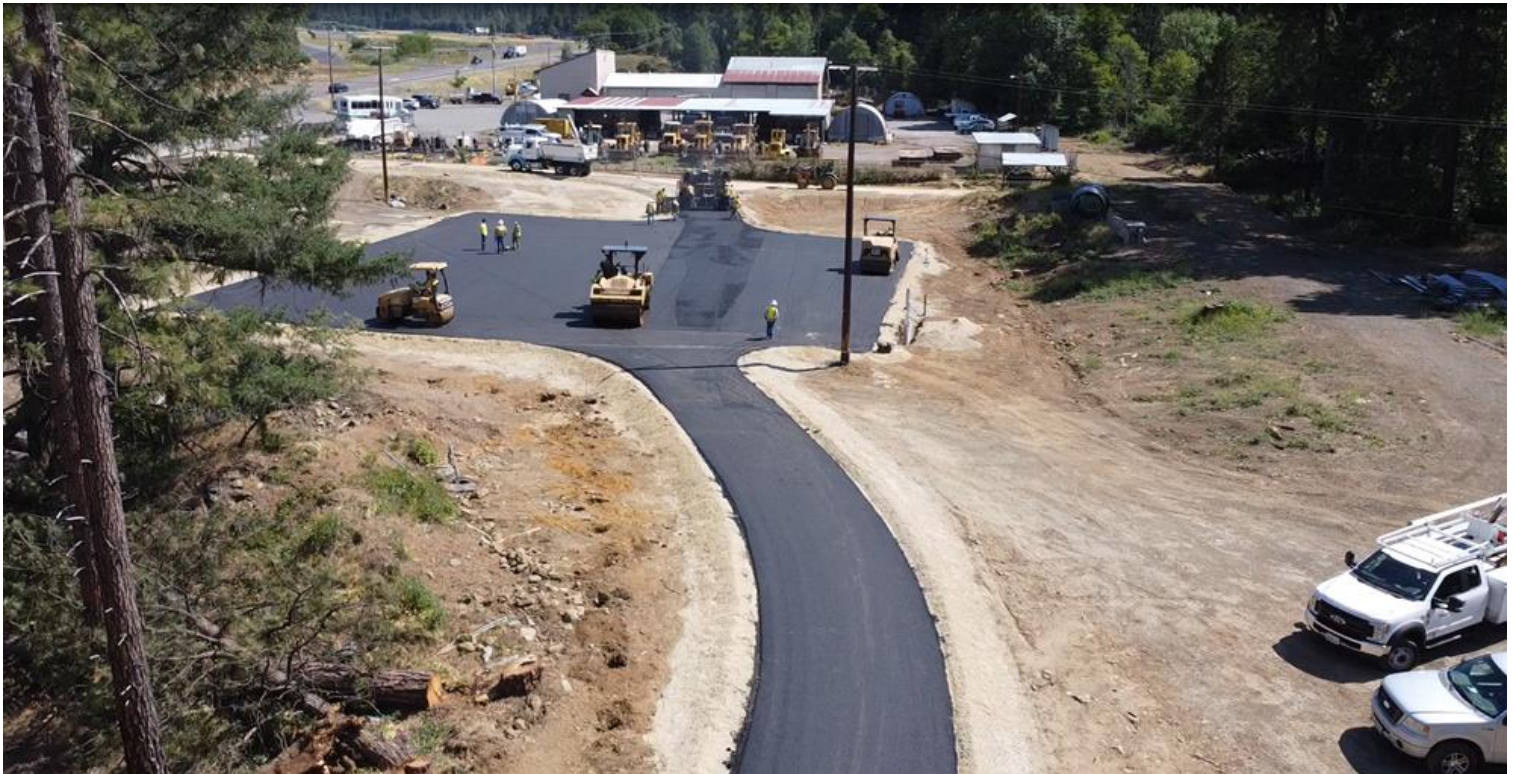
Paving operations (contractor) for the new Transit bus parking lot adjacent to Lance Gulch Road
