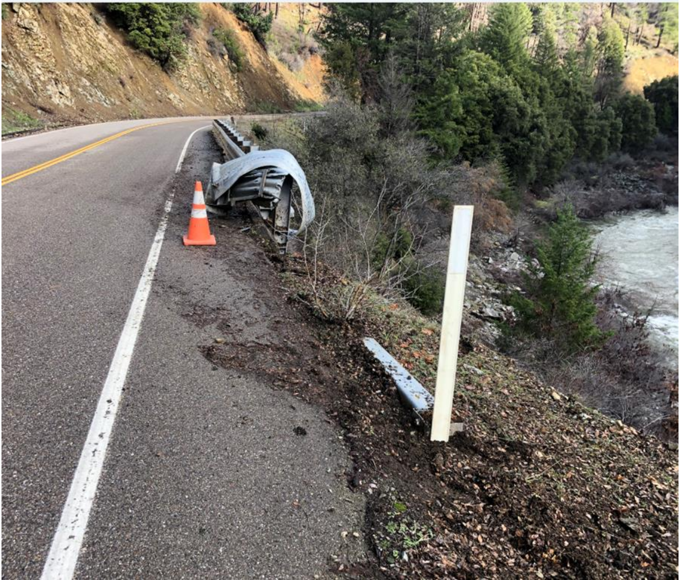
Damaged guardrail by an errant driver on Hyampom Road
