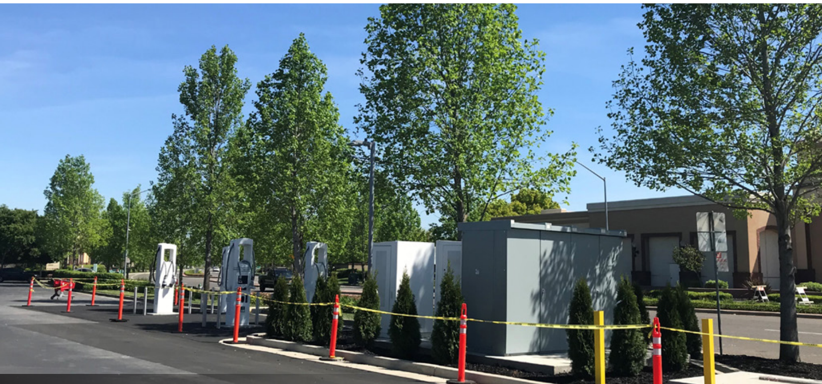
Images courtesy of Paired Power and Electrify America
