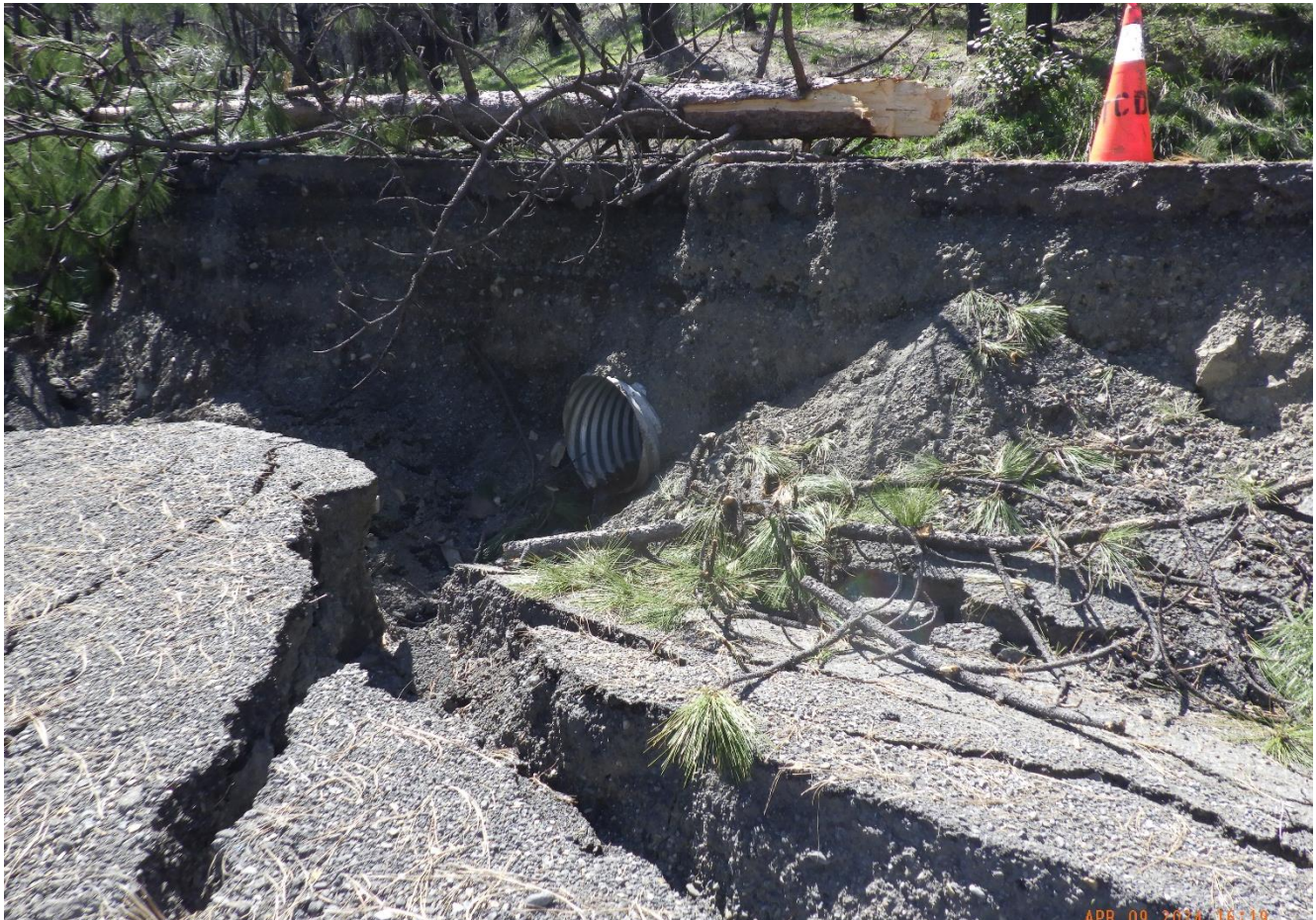
Ruth Zenia Road, late March road damage one of several locations at about Post Mile 18.75
