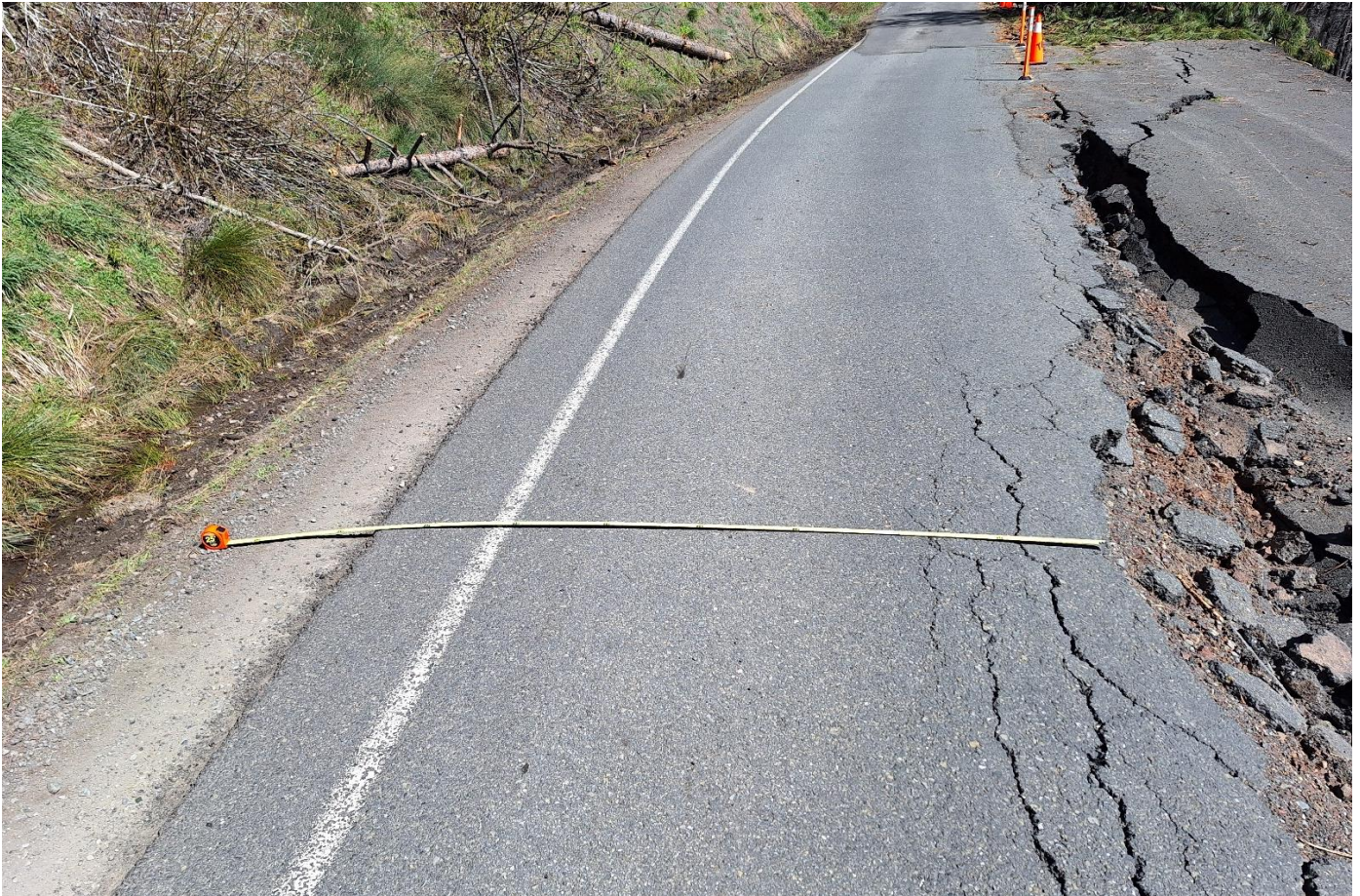
Ruth Zenia Road, late March road damage one of many locations at about Post Mile 18.75
