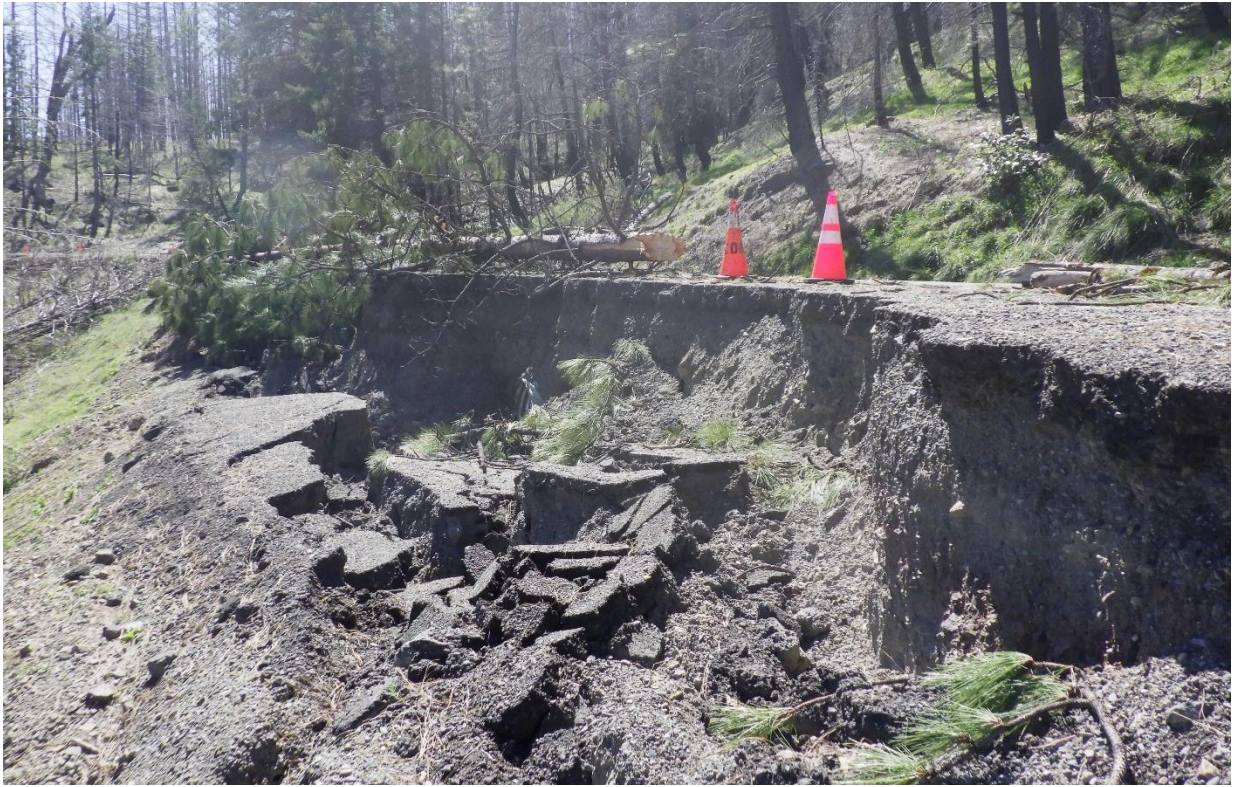
Extensive road damage
