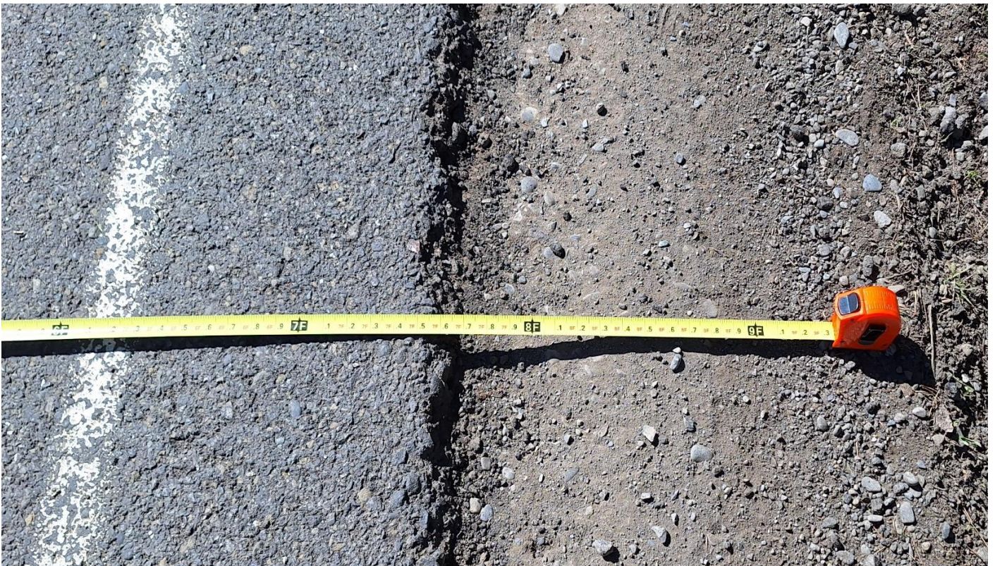
Only 7 ft-6 inches road remaining of the typical 12 ft wide lane
