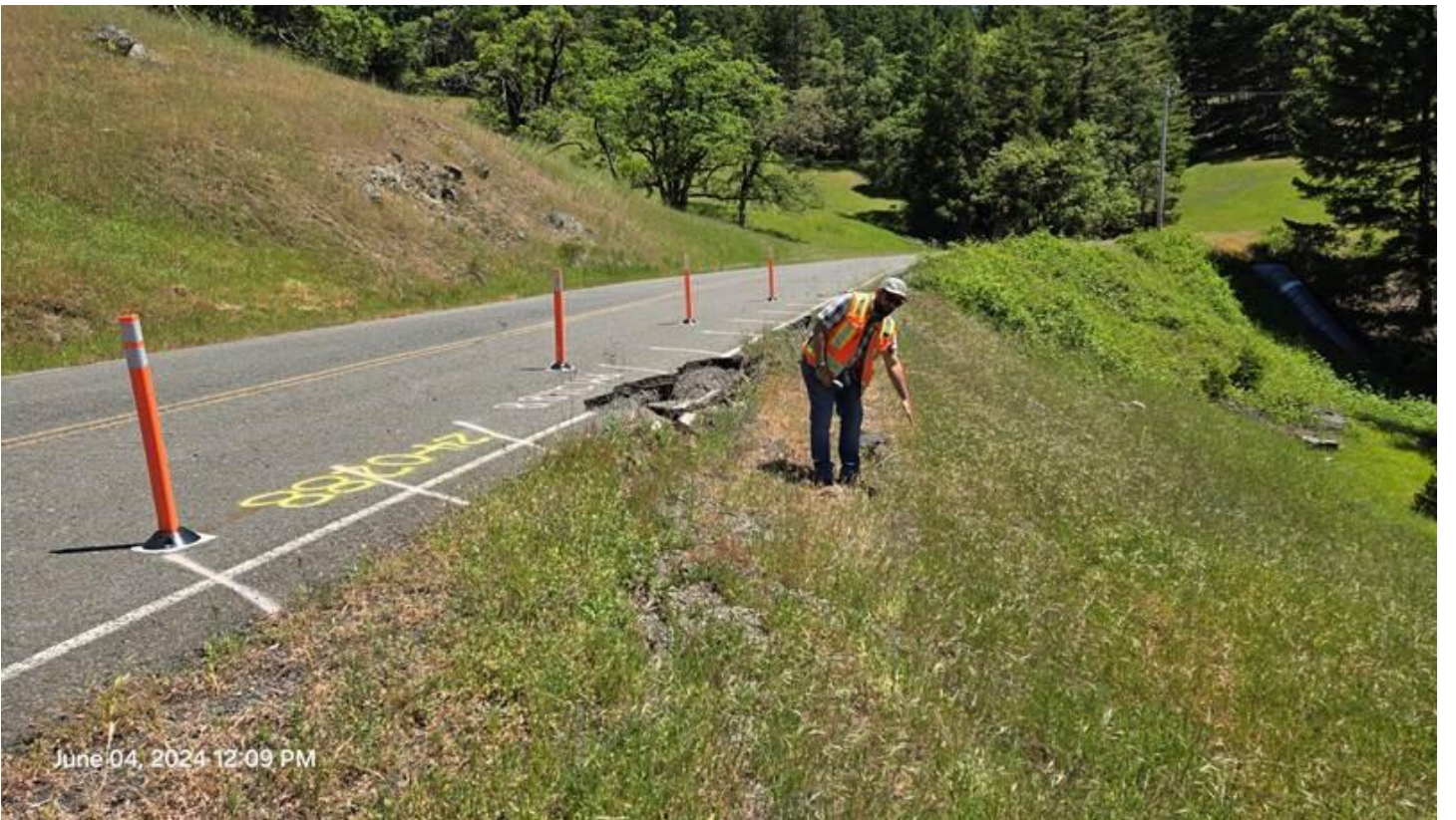
Storm Damage assessment Ruth-Zenia & Mad River Roads by engineering staff
