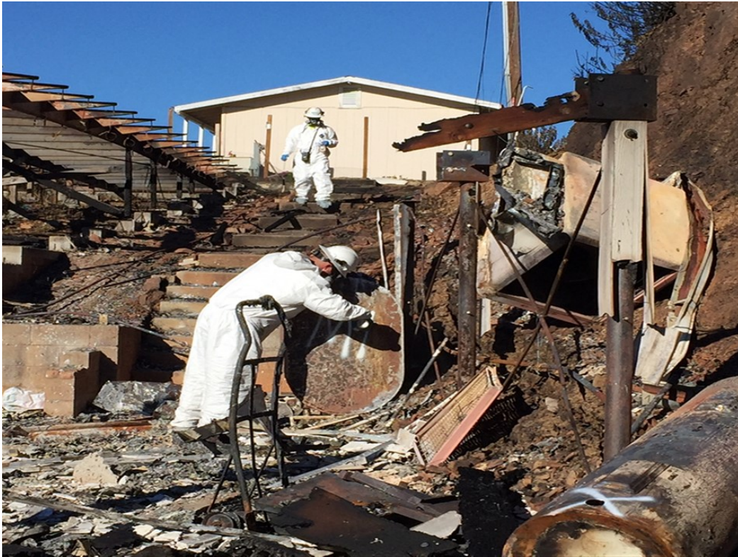
HazMat Crew marking the heating fuel tank with the letters “MT” to indicate contents have been removed and the tank is empty.
